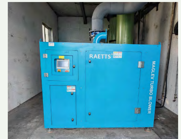
Supplier water treatment aeration equipment retrofits
